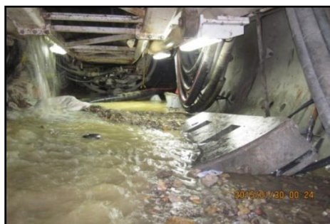
Fig. 3. Flow of fault zone mud and water towards the TBM cutterhead
